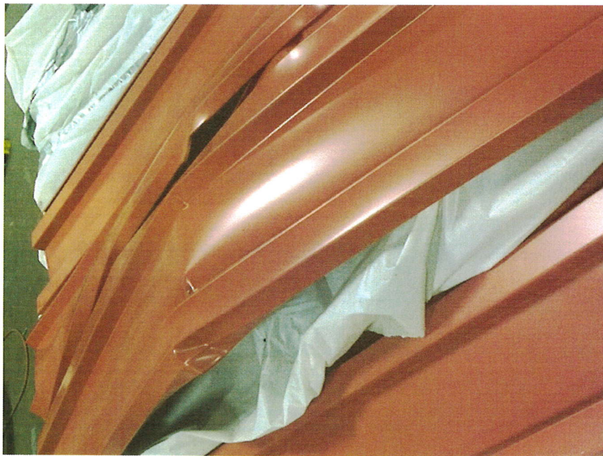
TYP. FAILED DISENGAGEMENT OF PANEL
